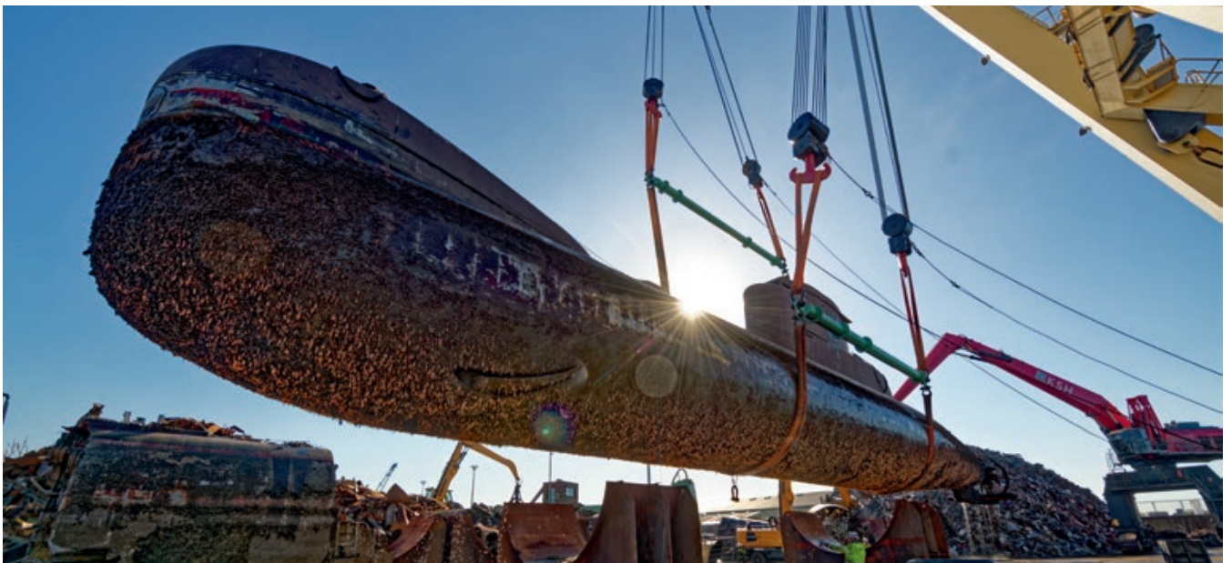
9.00 a.m.: The floating crane lowers the U 15 - which weighs some 450 tonnes - into the so-called cradle. Here, the submarine is kept stable until the hull is dismantled.
